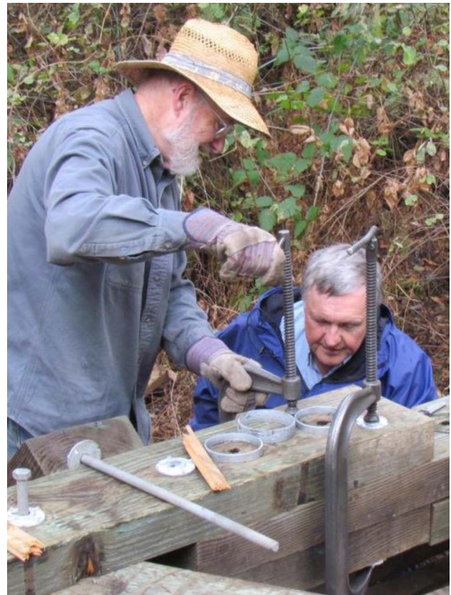
Charlie Right (bearded) and James Marshall working on a bridge join out in the brush.
